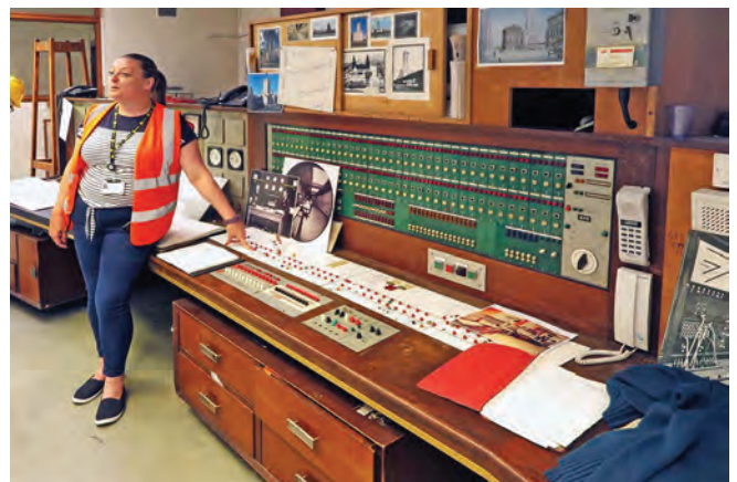
A closer look at the 1930s ventilation and control boards.
